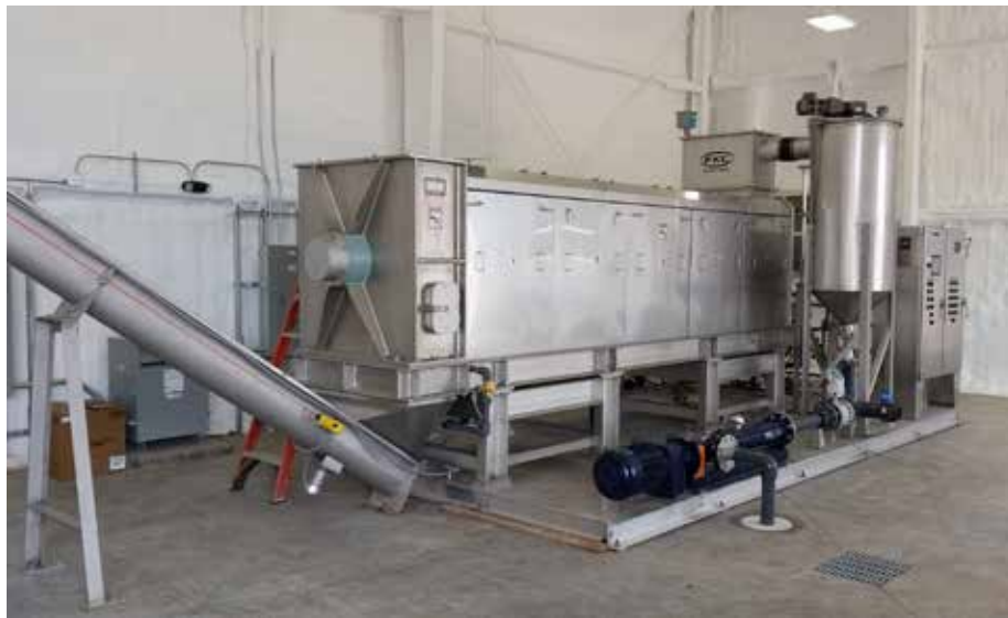
Sludge Dewatering Skid
