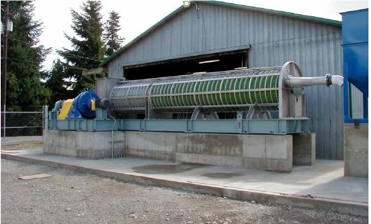
Septage dewatering screw press with a capacity of 6,000 gallons/hour
